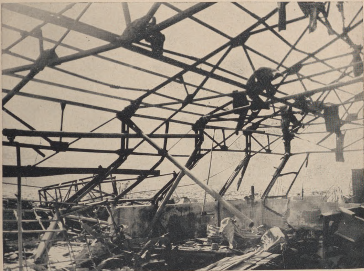
Figure 6.74. Light steel frame industrial building, 600 yards from ground zero in Japan. The roof and wall sheathing was stripped by the blast, and the combustible contents destroyed by fire.
