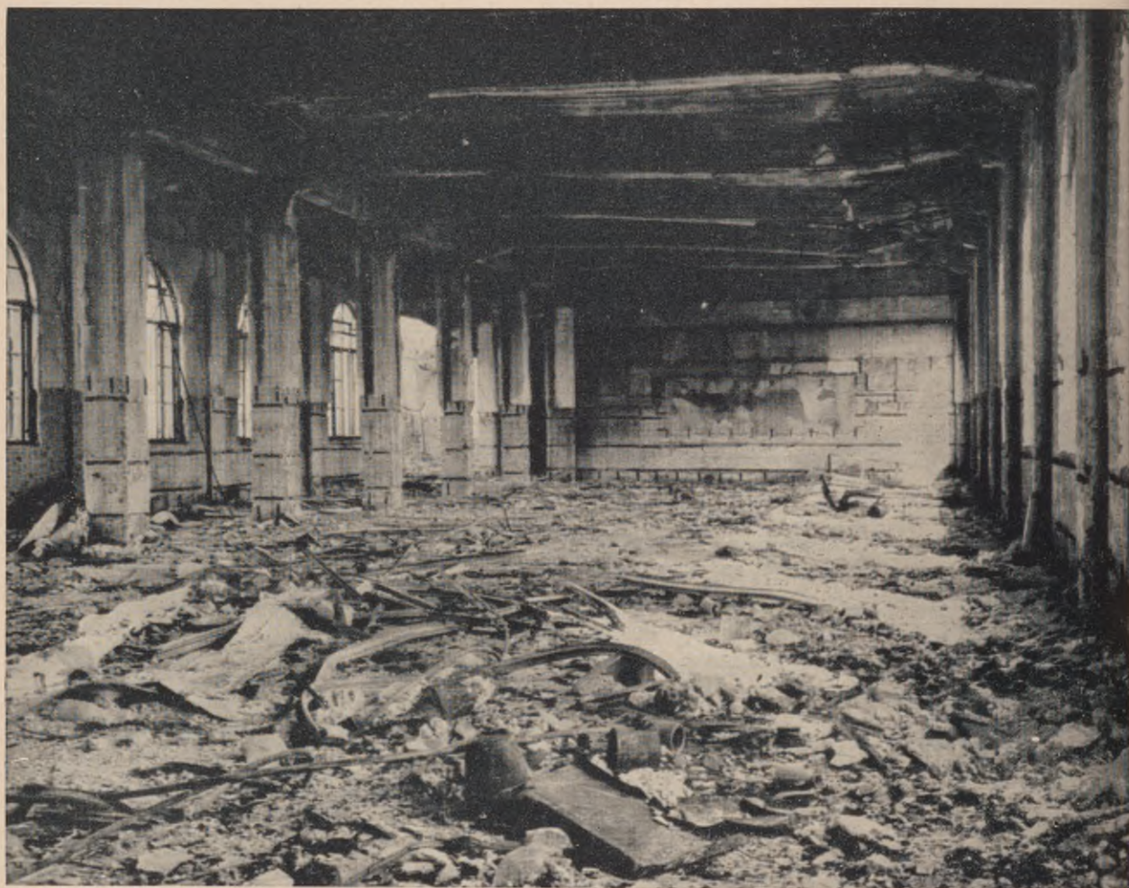
Figure 6.71. Reinforced concrete building, 240 yards from ground zero in Japan. The walls are intact although the interior was destroyed by fire.
