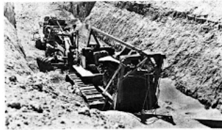
Figure 12.4c: Earth-moving equipment protected in deep trench at right angles to blast wave motion (30 psi overpressure).
